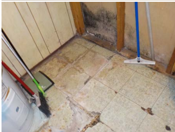
fungal growth in laundry
