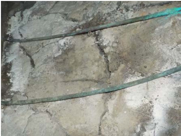
oil fuel lines in crawl space
