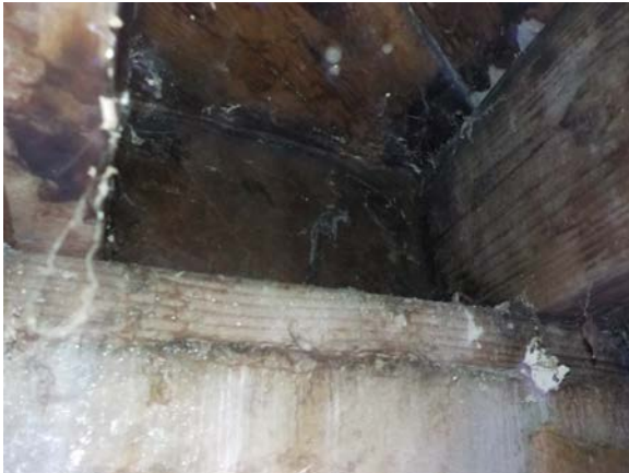
rot under shower
