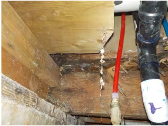
rot on joist under tub
