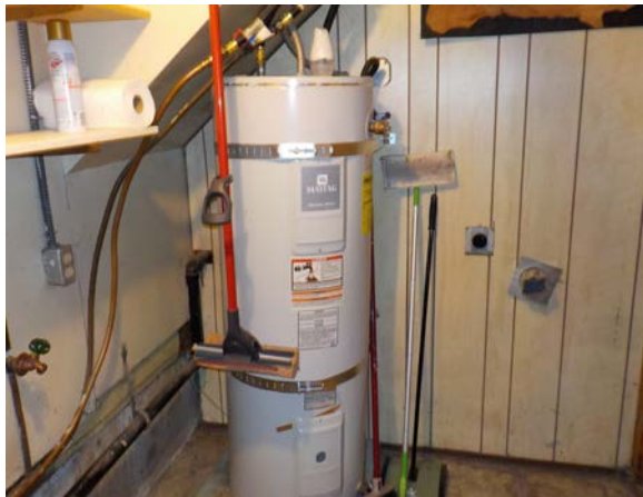
hot water heater
