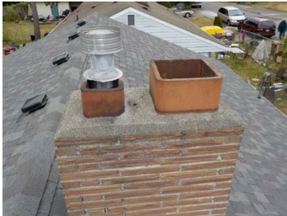
Chimney caps needed
