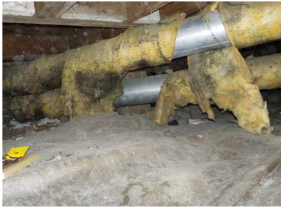
crawl space ductwork
