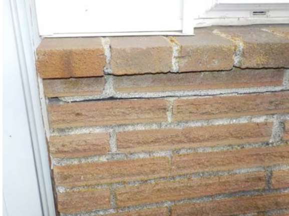
front brick settling
