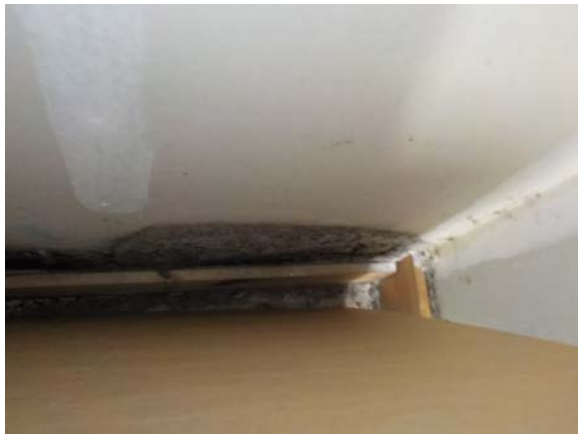
fungal growth in garage
